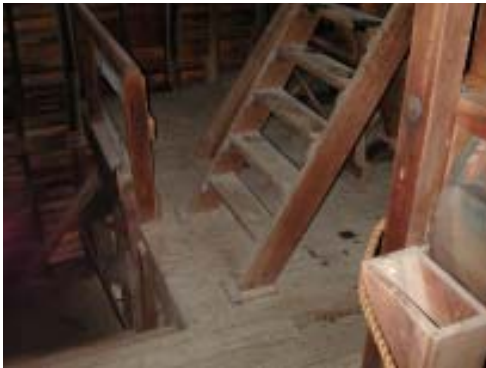
A stairwell behind the reader could present a safety problem.
